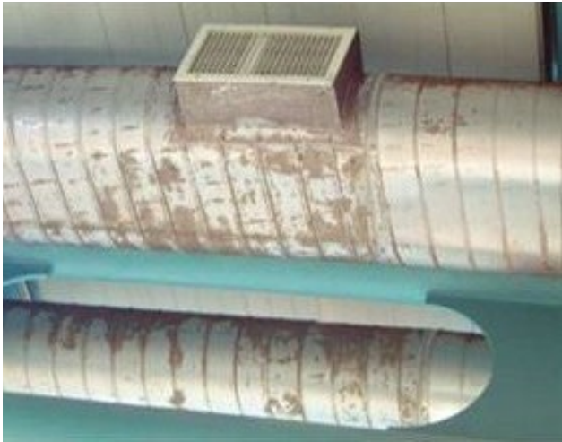
Corroded Air Handling System
